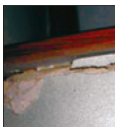
Building damage by moisture
